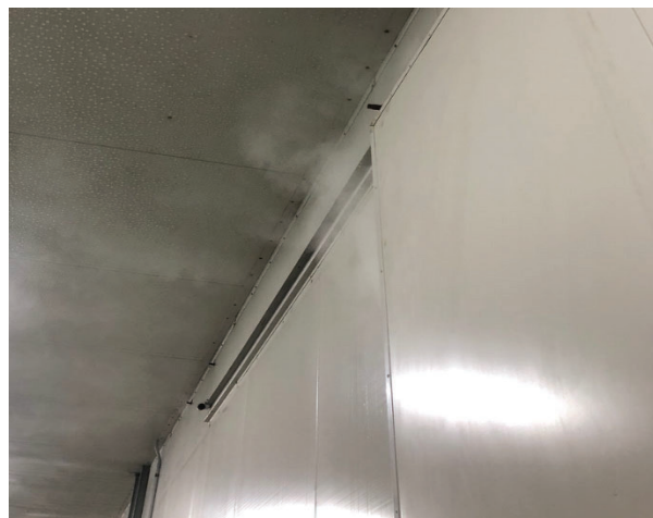
Figure 1 Steam escaping through inadequate door seals. Image: Judy Allan
