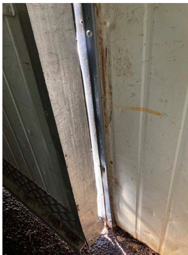
Figure 1. Damaged door frames give poor physical exclusion.
