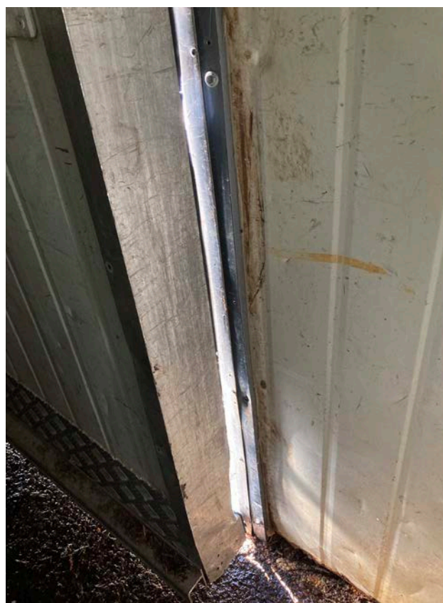
Figure 1. Damaged door frames give poor physical exclusion.
