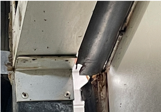
Figure 4. Damaged door seals prevent effective exclusion. Image: J Allan
